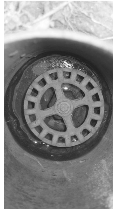
Figure 27 - Water in Valve Box
