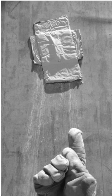
Figure 25 – Storage Tank Leak
