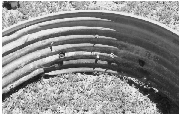
Figure 24 – Prior Repairs to Drinker
